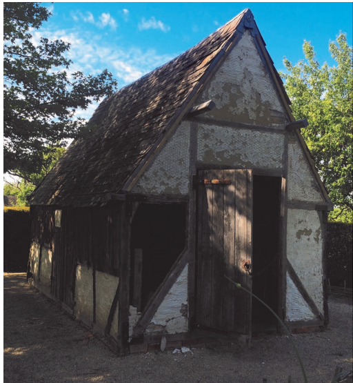
The Forge is a great teaching tool for the schools teams, and is much in need of repairs—starting with the roof. The Trustees have agreed that the current roof must be replaced with wooden shingles.
